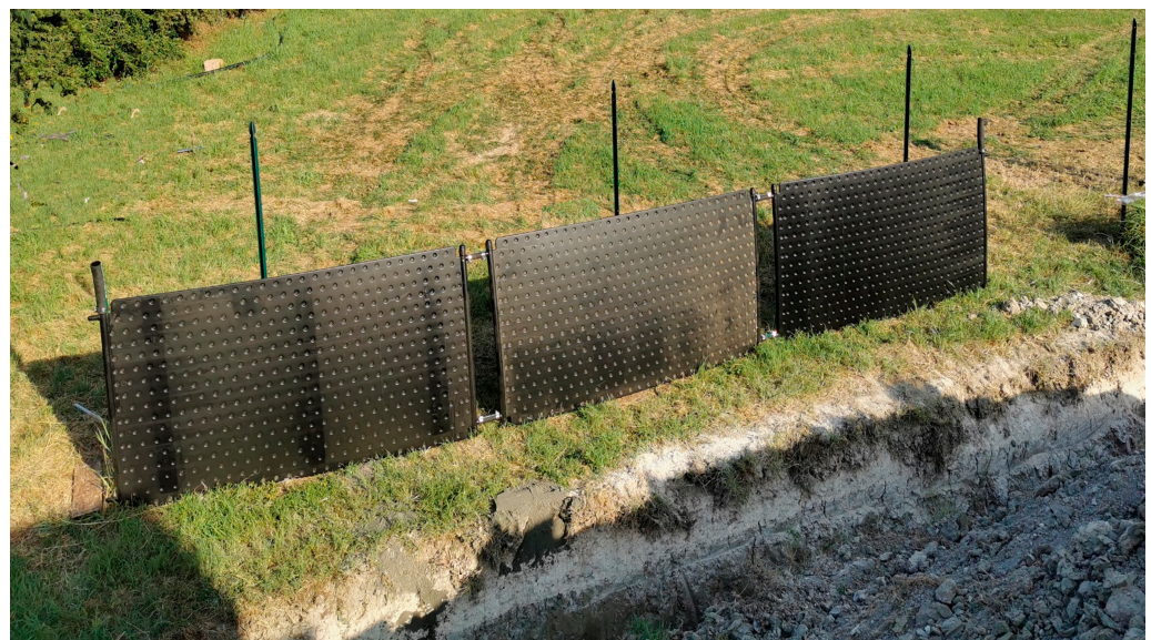
Figure 1. A geothermal line composed of 3 FPs before to be installed in the trench at the TekneHub laboratory of UNIFE.
