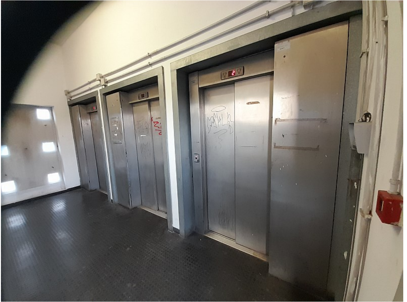
Figure 7 - Example of lack of cleanliness at Anagnina underground station in Rome
