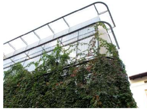
Fig.3 – Vegetal screen on structural glass curtain wall in an office building in Cologne
