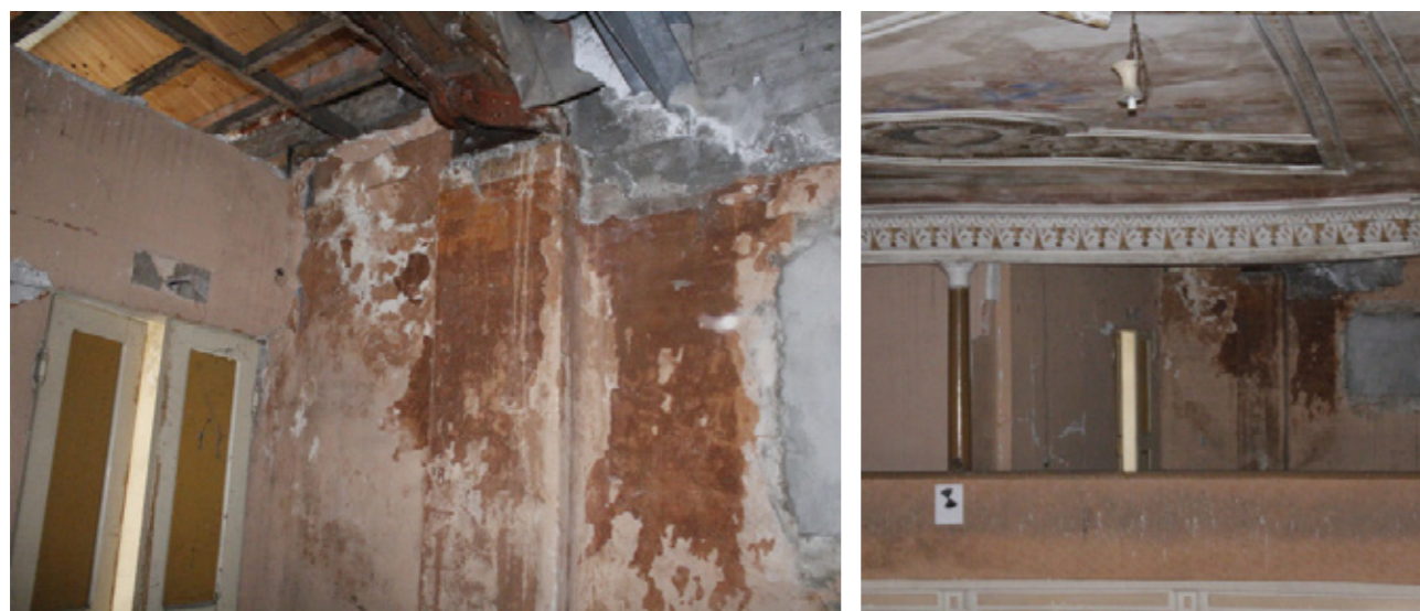
Fig. 98- 99- 100 Reflectance analysis of the hall. The northwest sector of the 3rd order of boxes. The interpretation of the data is described in paragraph 5.2.2.5. Developed by M.Suppa
