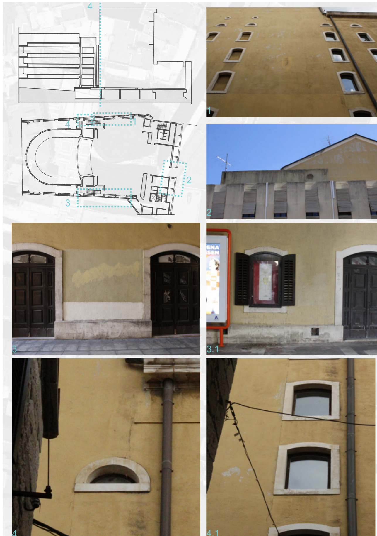
Fig.38 - views of the principal morphologies of decay present along the exterior facades of the Split Theater. Views 4 and 4.1 show a lesion running along the east fornix located between the stage area and the cavea Developed by M. Suppa
