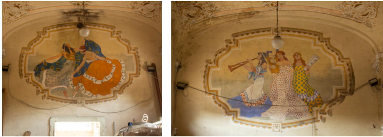
Fig. 65-66 Novi, Teatro Sociale, interior decoration of the entrance hall. Photographic survey dated July 2020. Ph M. Suppa.
