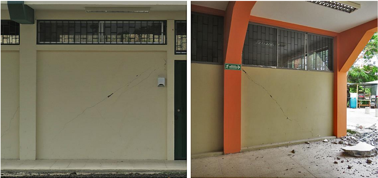
Fig. 2 Masonry infills displaying DS 1 damage state observed after the Ecuador 2016 earthquake (photos by E. Miranda).
