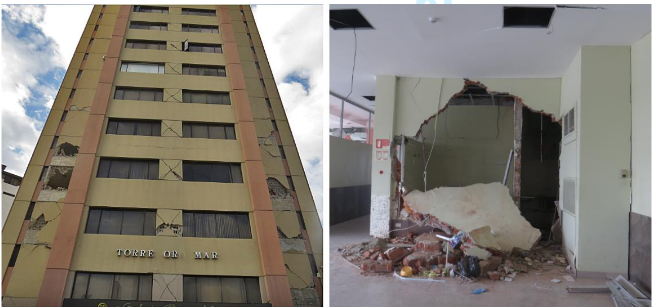
Fig. 1 Masonry infills damaged after the Ecuador 2016 earthquake (photos by E. Miranda).
