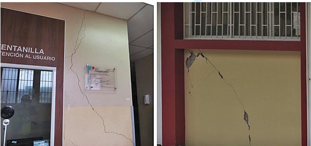
Fig. 3 Masonry infills displaying DS 2 damage state observed after the Ecuador 2016 earthquake (photos by E. Miranda).
