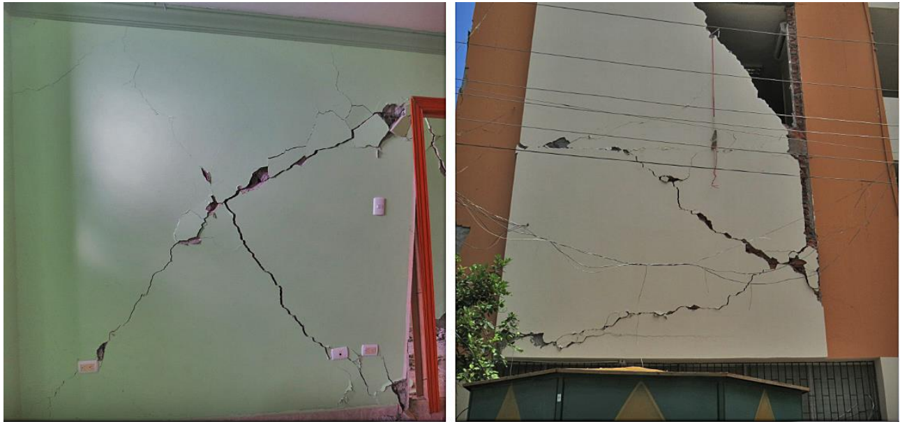
Fig. 4 Masonry infills displaying a DS 3 damage observed after the Ecuador 2016 earthquake (photos by E. Miranda).
